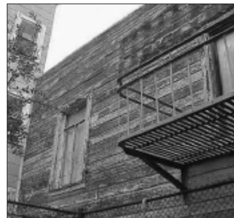
Figure 7. Before correction of peeling paint
